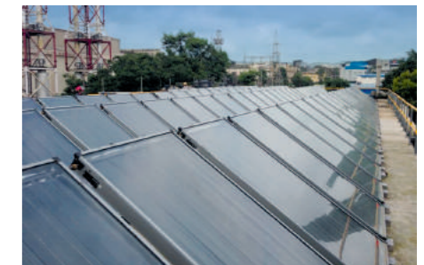
Rooftop solar array at Thane
